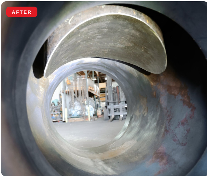
Inside the modified valve: the machined arc conduit guide (upper crescent) blends into the bore so the pig passes without a step.
